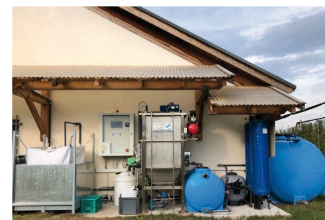
Physical-chemical wastewater treatment system
