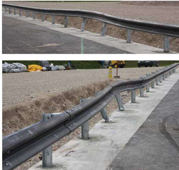
Damage to the device
