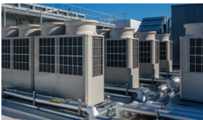
HVAC and cooling equipment
