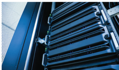
Cabinets, racks, shelving and accessories
