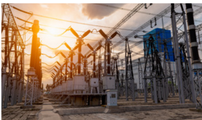
Generators, switchgear and transformers
