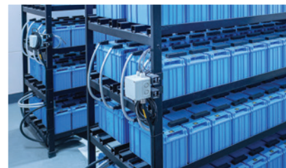
Battery energy storage systems (BESS)
