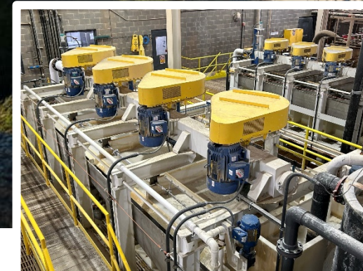
Images (top to bottom): Newly installed 100ft clarifier at Schoolhouse Plant, newly installed flotation capacity at Schoolhouse Plant
